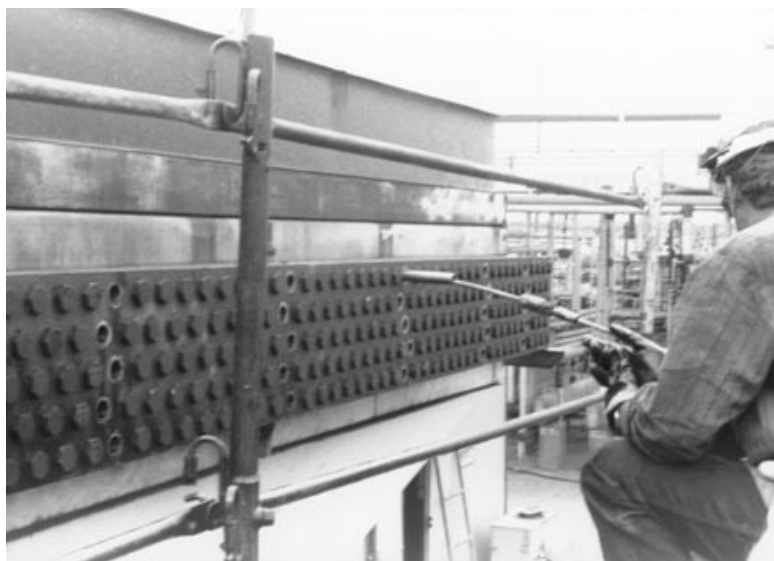
Figure 3. Field data acquisition for finfan MFL inspection. Note the conduit inserted into the outside tubesheet that allows for the probe to enter the tube, starting at the second (internal) tubesheet
