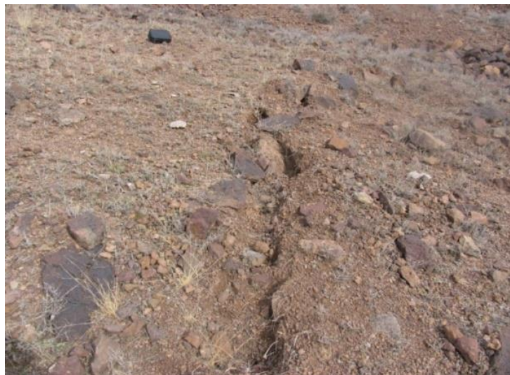
Figure 2. II-nd rupture crackorder in the landslide area
