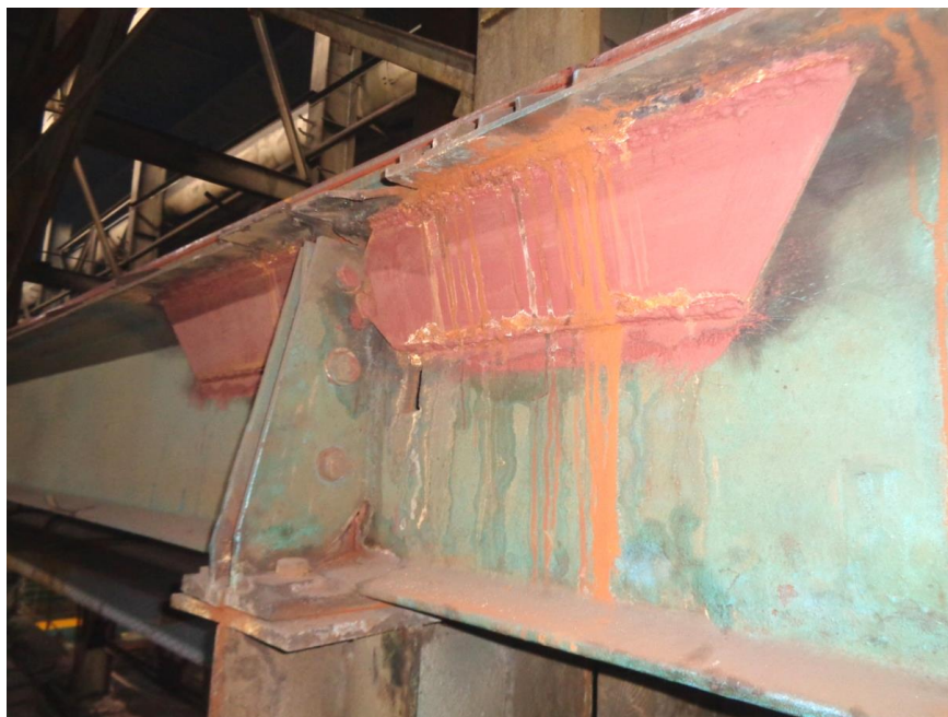
Figure 3. Reinforcement of crane beams with cracks by lamellas
