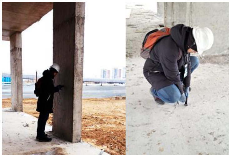
Picture 1. Assessment of the technical condition of monolithic floor slabs and pylons
