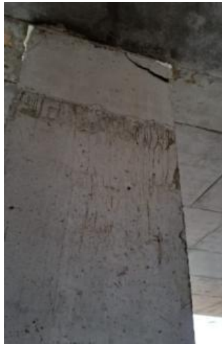
Picture 3. Spalling of concrete in the connection area with the floor slab
