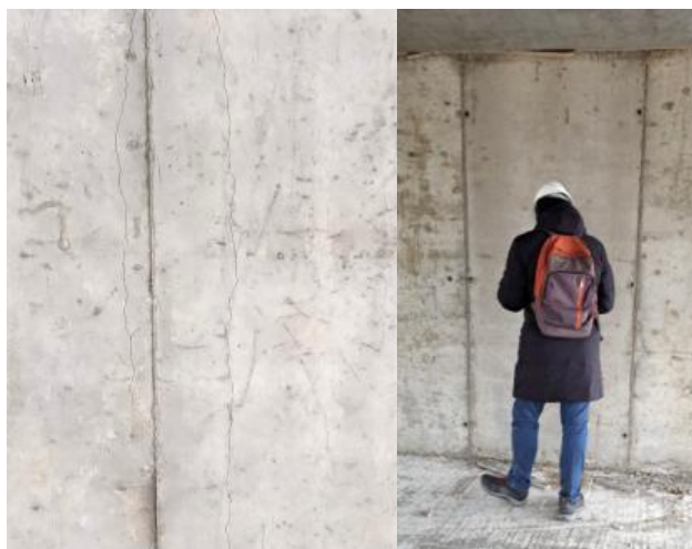
Picture 2. Longitudinal crack, opening 0.2 mm in size
