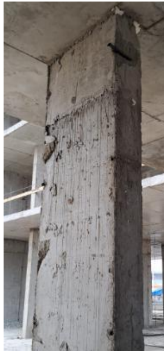
Picture 4. Violation of the thickness of the protective layer of concrete with the exposure of reinforcement
